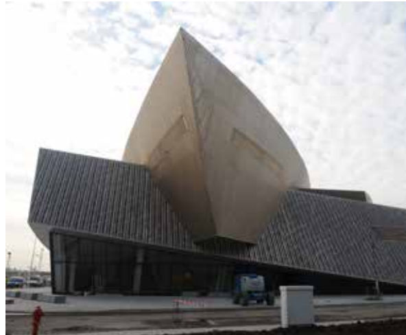
Construction of the Congress Centre in Mons on the "Ateliers SNCB" site rehabilitated by SPAQ∞E
