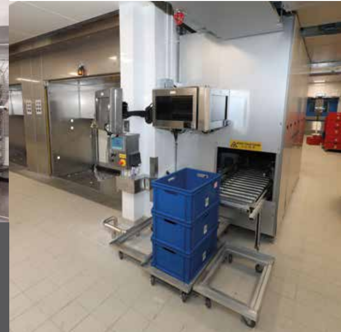
SPACE TOWER forms an integral part of the production process.
