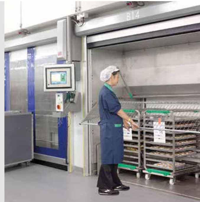
Typical array of temperature controlled Trolley Towers.
